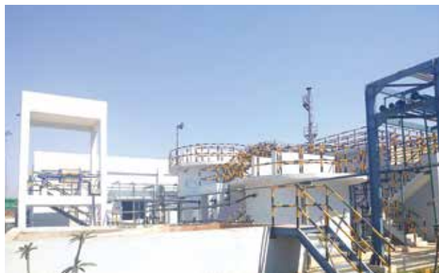
▶ Zero Liquid Discharge at Goindwal Plant
